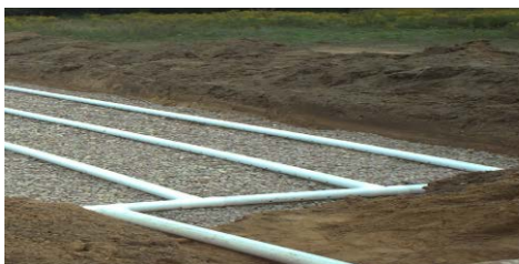
Figure 3: An example of the closed loop system found in an absorption bed.
