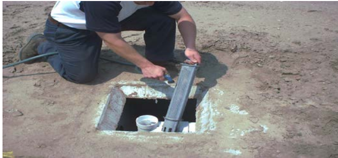
Figure 2: Hosing an effluent filter off into the septic tank
